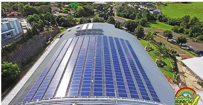
FIGURE 4: LISMORE CITY COUNCIL'S 100 kW SOLAR ON GSAC
